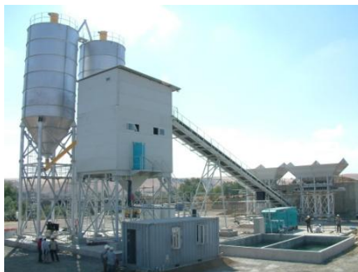
1个2.33立方米搅拌站 1X2.33 cubic meter Stationary plant
