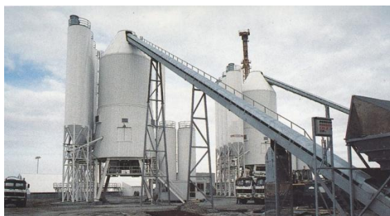
2个3立方米塔楼式搅拌楼 2X3 cubic meter Tower plant
